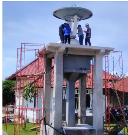
Fig. 2.2.1.1. The SATRAK 550 Antenna in IMRO Ground Station
